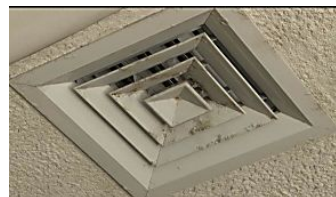
Ventilation system concerns at UH laboratory building
